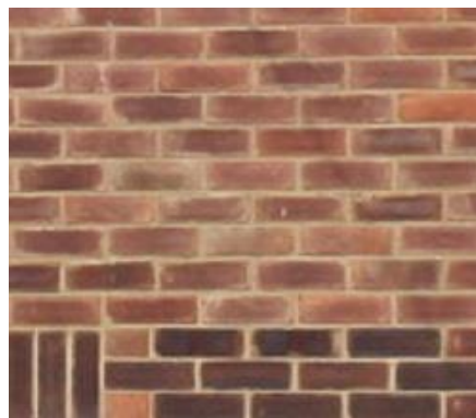
Fig. 9 Brickwork on a house of the third quarter of the 20 th century
