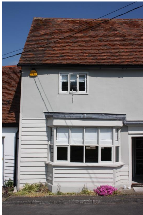
Fig. 1 Render above weatherboarding on Wingtons
