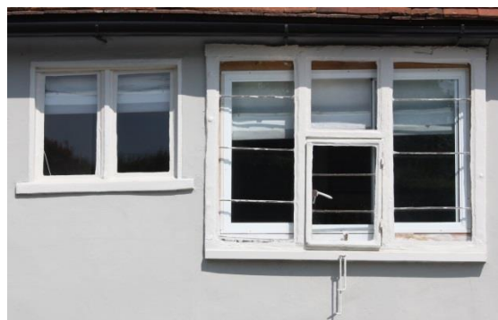
Fig. 15 Early 17 th -century mullion window to left of 18 th -century casement window
