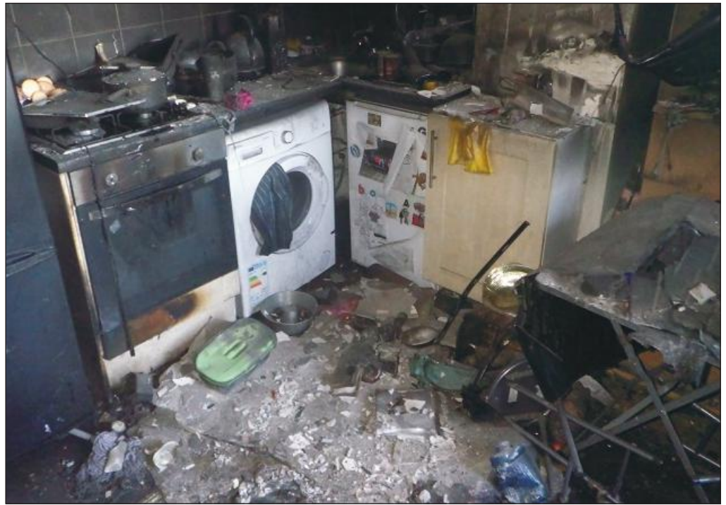
The damage caused to one flat after a scooter caught fire while being charged in a bedroom
